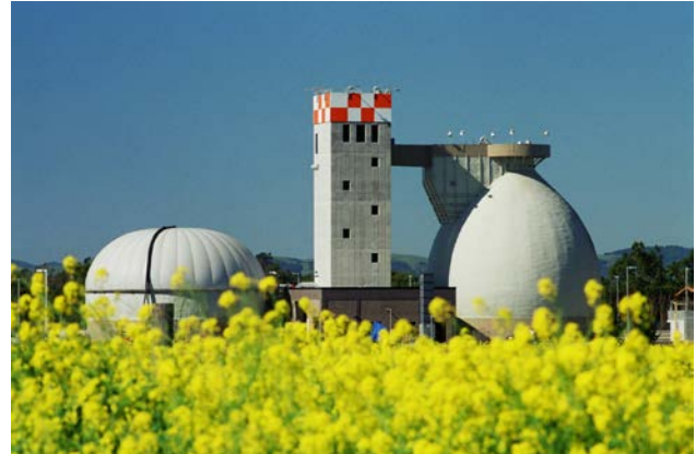
Treatment plant biogas holder (left) and digester (right)
