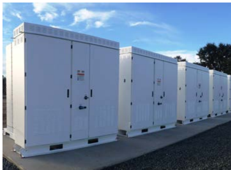
Stationary storage batteries used to store energy during the night for use during the day, decreasing energy demand charges
