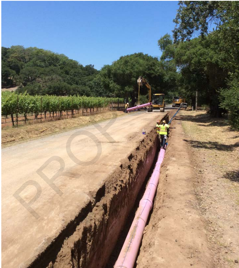
Installation of recycled water pipeline in the Los Carneros Water District area
