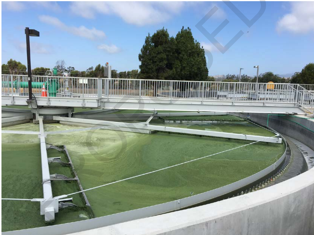
Dissolved air floatation (DAF) clarifier, Soscol Water Recycling Facility
