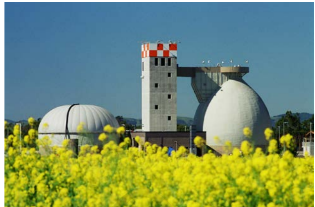
Treatment plant biogas holder (left) and digester (right)
