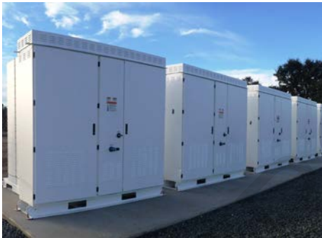
Stationary storage batteries used to store energy during the night for use during the day, decreasing energy demand charges
