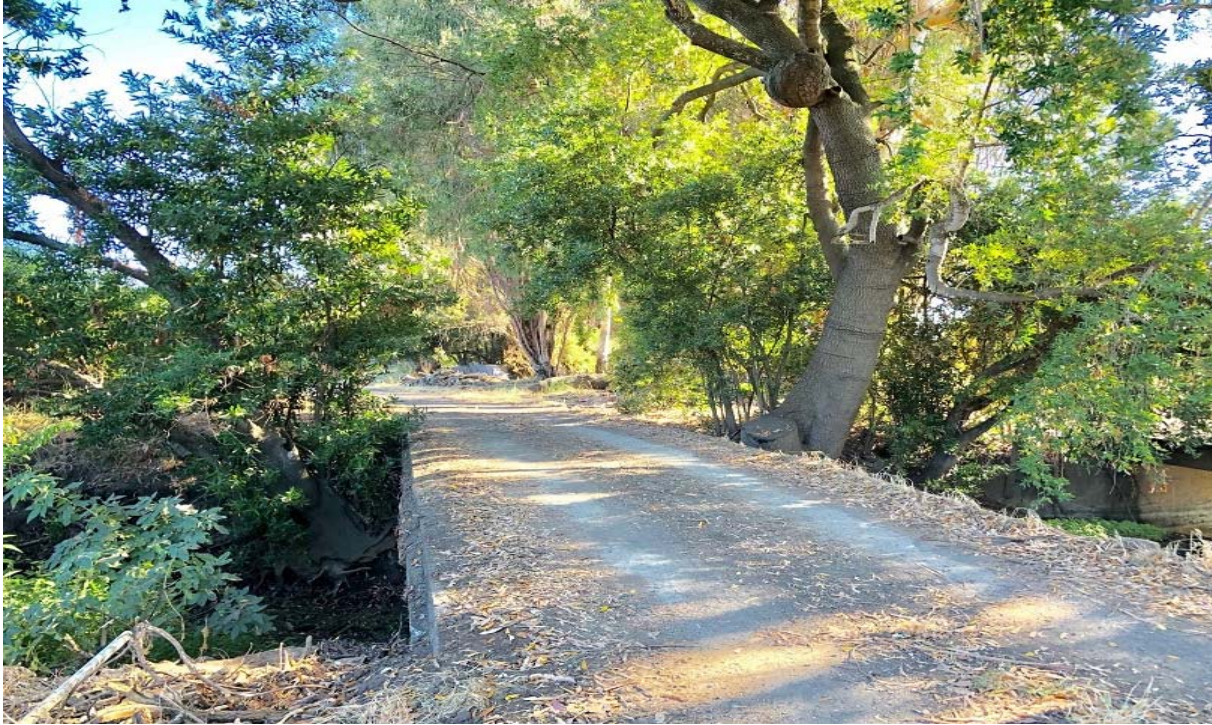
Photo 11: Facing south. Bridge over Suscol Creek connecting access road to parcel (July 17, 2019).
