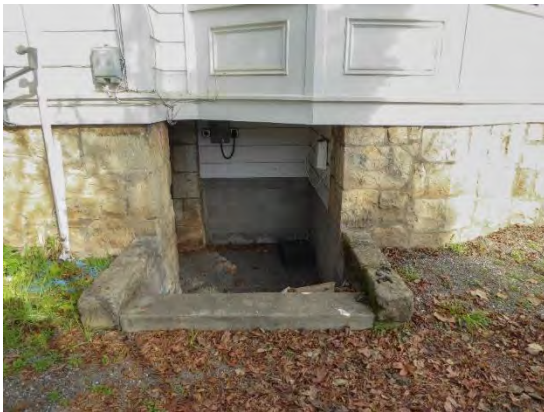
Figure 24: Masonry step down to side basement entrance at southwest façade. Looking northeast.
