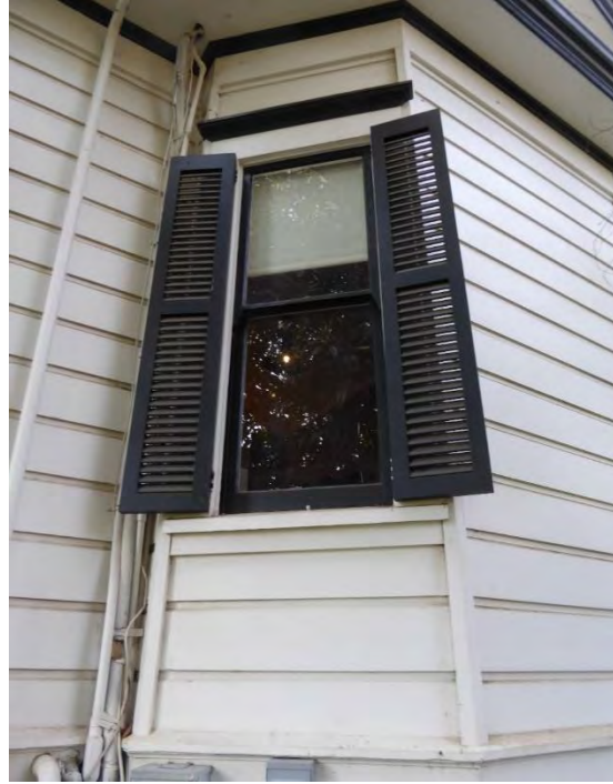
Figure 16: One of two standard windows within angled projecting bay at northeast façade. Looking west.
