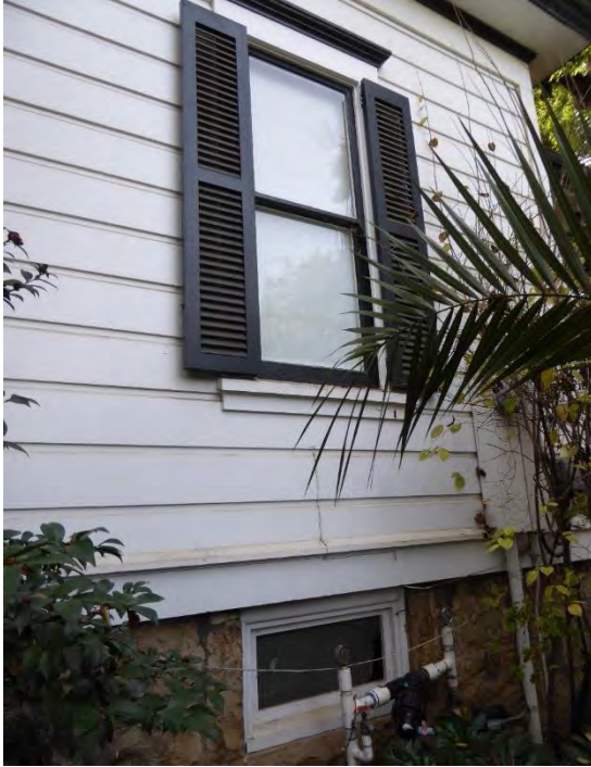
Figure 15: Standard window at north end of northeast façade with non-original shutters. Looking west.
