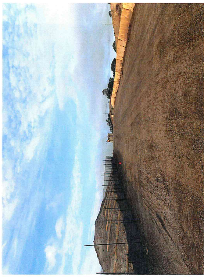
Landfill ramp, litter fence and K-rail for customer and employee safety
