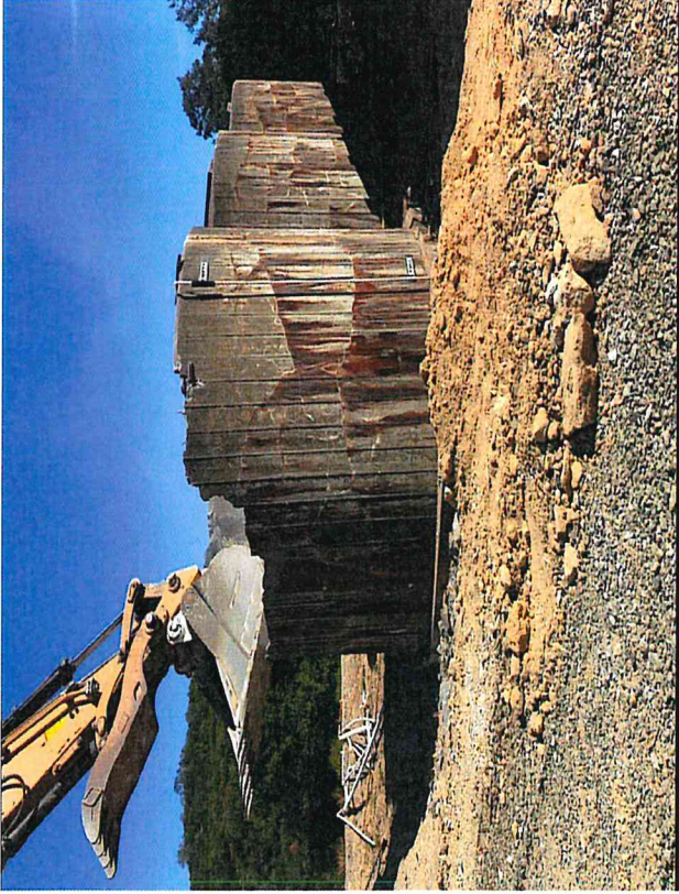
Demolition of three concrete leachate 10k gallon tanks with 30k gallon capacity
