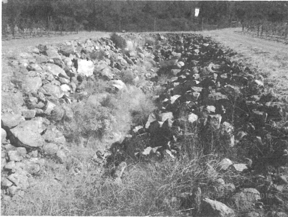
Photo 3. Upper portion of unnamed intermittent stream that was channelized (looking upstream).
