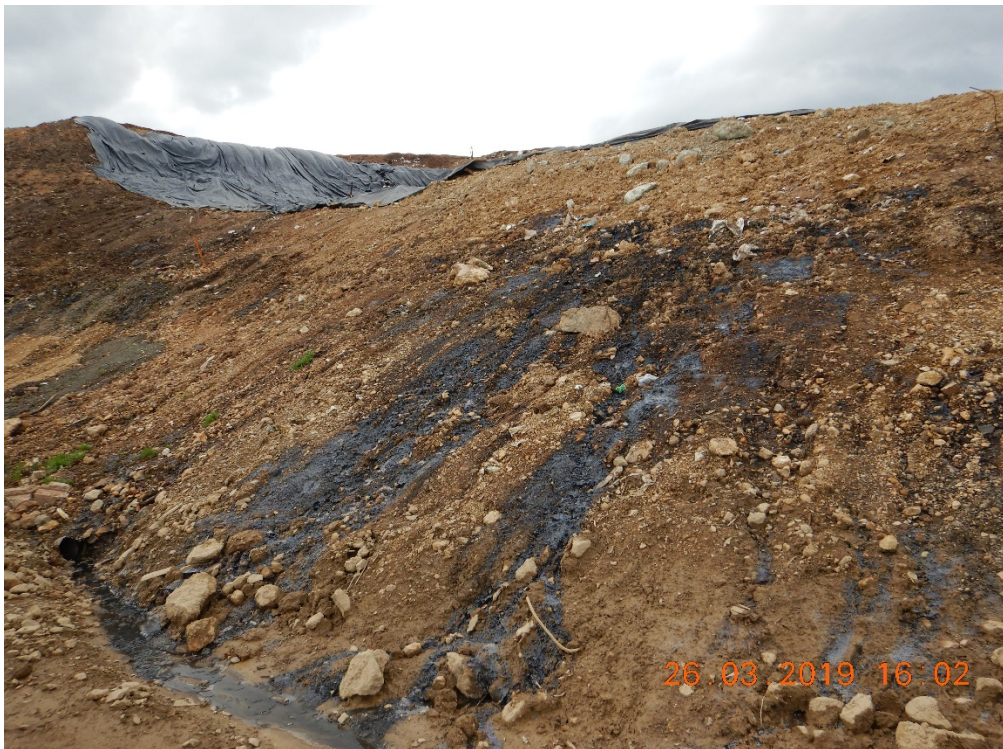
Photo 684- active leachate seeps draining into the drop inlet, looking northwest
