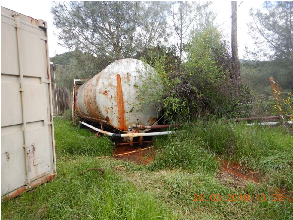
Photo 521- rust staining and leakage from the leachate condensate tank, looking northeast.
