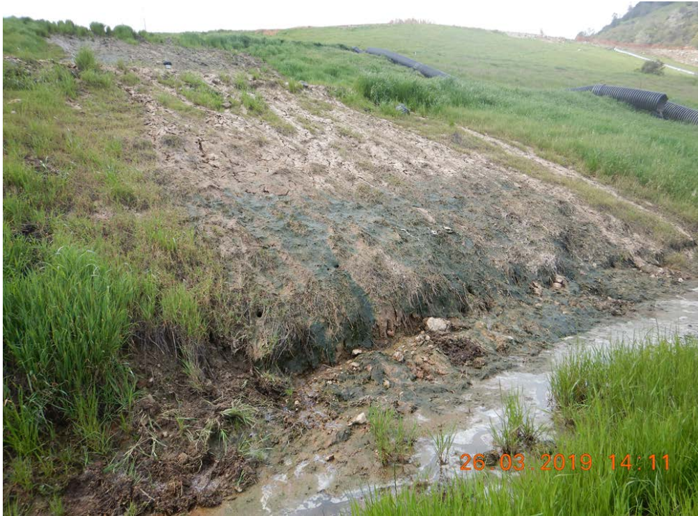
Photo 615- erosion from stormwater and leachate overflow, leachate ponding on the bench, looking northwest.
