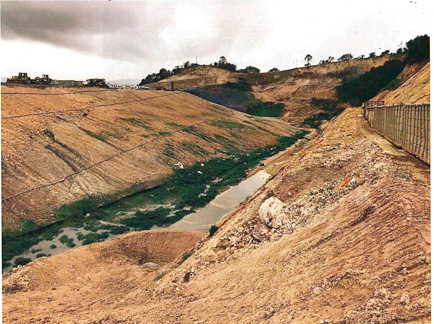
Exhibit 6 - module 5B drainage 4-2-19
