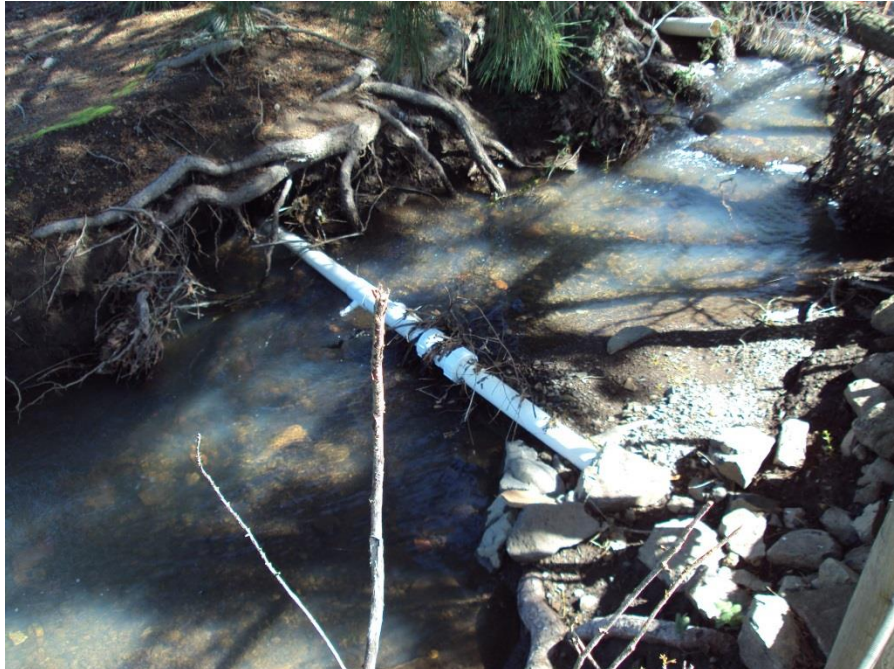
Photograph 48: Easterly view of water line crossing the blue line stream. March 17, 2016
