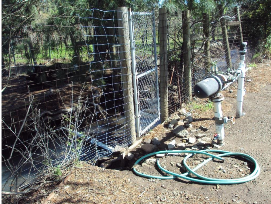
Photograph 47: Easterly view of water line crossing the blue line stream and of water valve and filter. March 17, 2016
