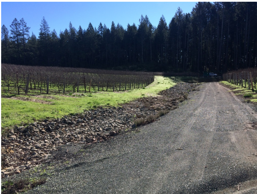
Photograph 18: South southeasterly panoramic view of rock lined swale, gravel access road and vineyard. January 26, 2016
