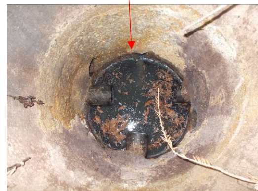
D-box for leach field
