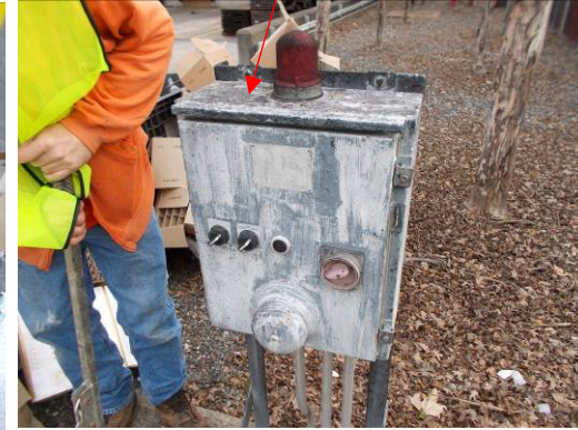
Control panel weathered.
