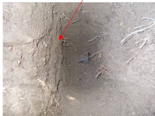
32" of soil cover over pipe
