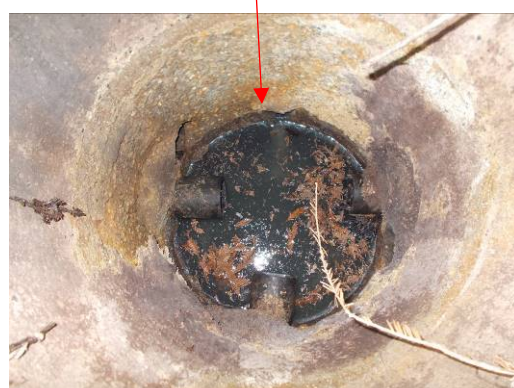
D-box for leach field
