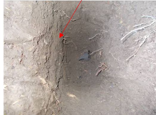
32" of soil cover over pipe
