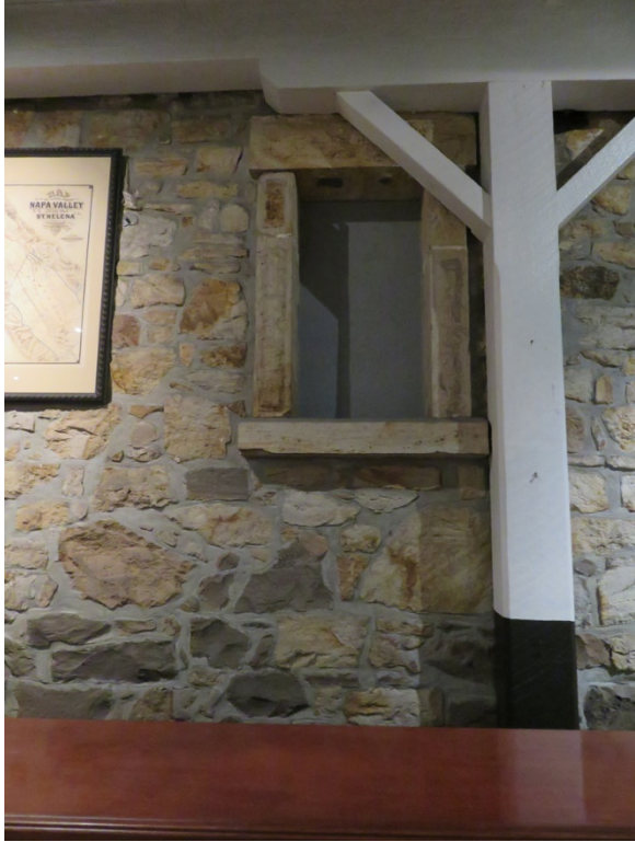
Tasting room, rear of Room A – note window infill and original timber structure.
