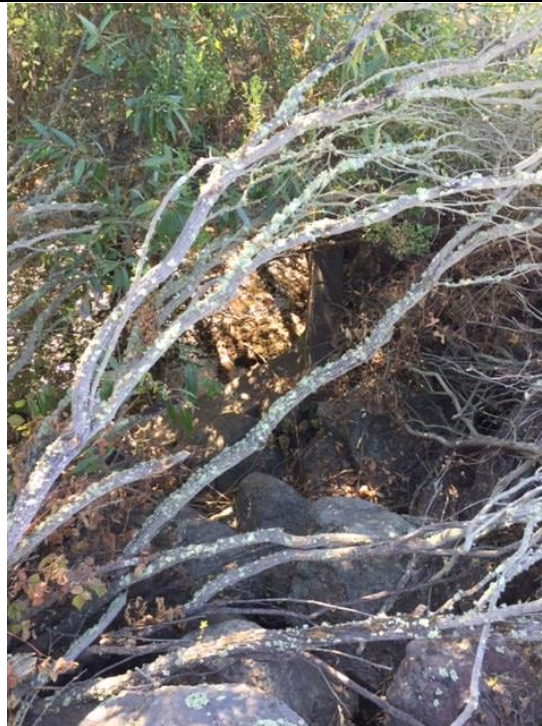
Photo 6: View of outlet of Sheehy Creek under Devlin Road on the western edge of the study area.
