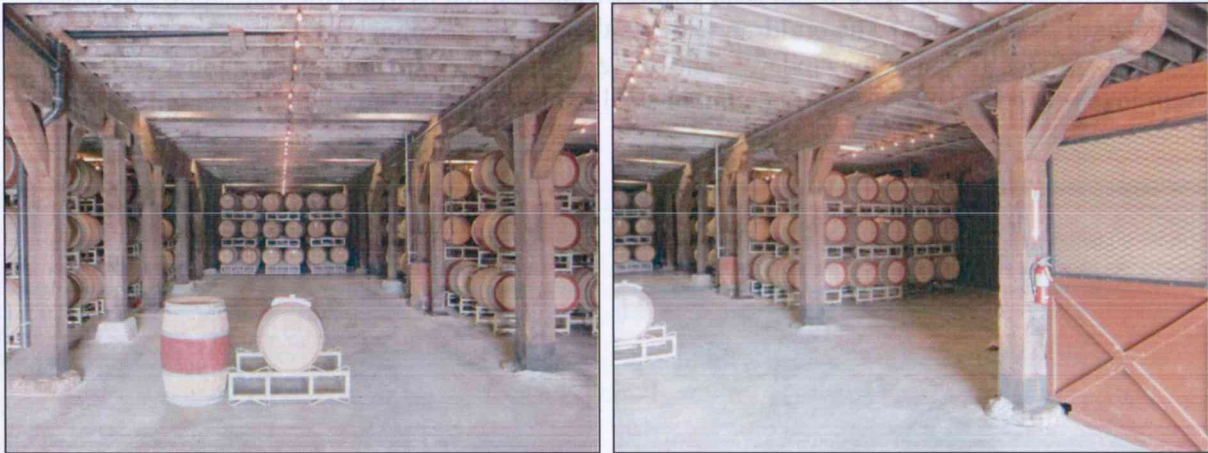
Figures 19 and 20. Left image shows the ground floor interior looking east from just inside the entrance. Right image details the timber supports of the ground floor interior.
