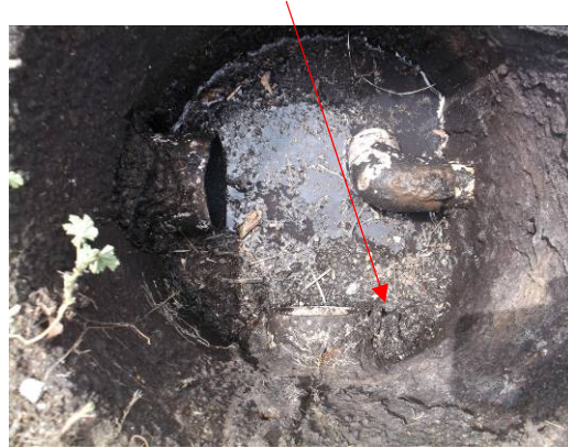
Distribution box. Soil debris.
