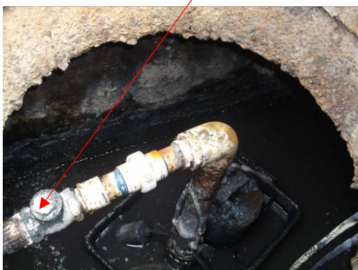
Erosion on fittings. Pump in plastic basin.
