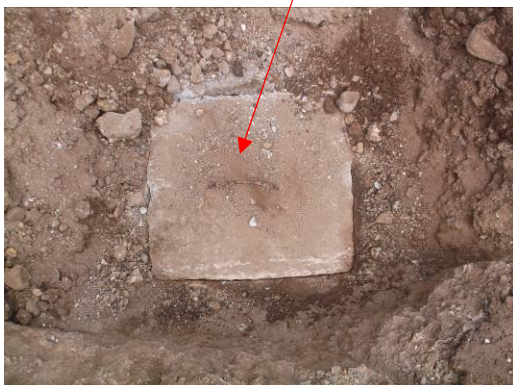
Septic tank lid. 12" of soil cover.
