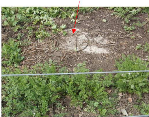
Distribution box no soil cover.
