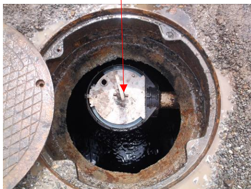
PW tank. Outlet filter.
