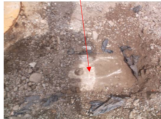
Electric box marked "water".
