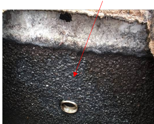
Erosion at interior of PW tank.
