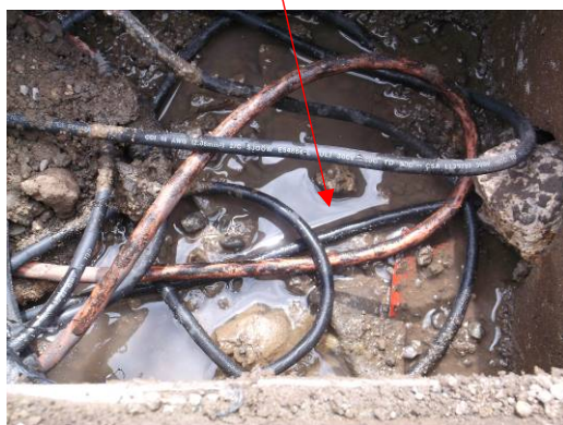
Electrical box. Wires standing in water.
