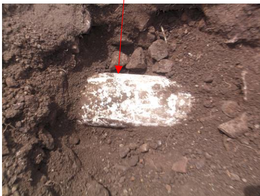
3" Hancore PVC leach line.
