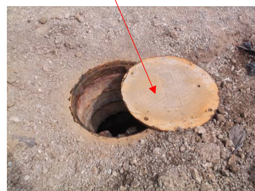
Metal riser and lid.
