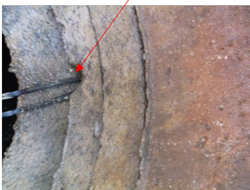
Penetration point not water tight.
