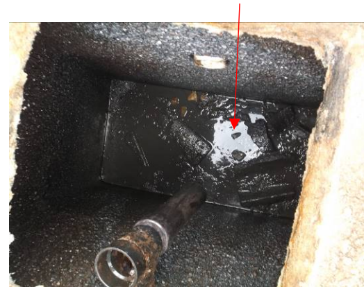
Debris in bottom of PW tank outlet.
