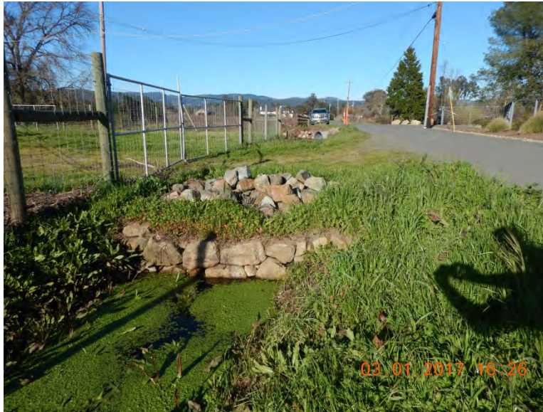
Photo 3: Vineyard Road Culvert at roadside ditch, north side of S. Whitehall Lane
