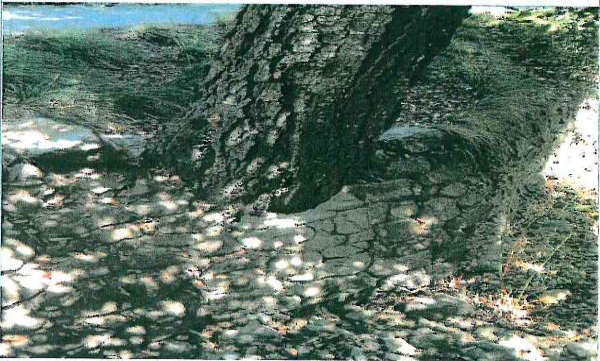
Photograph 12: Teal Creek river-rock banks with tree and erosion
