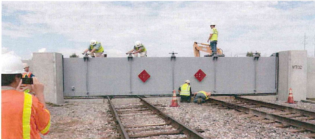
Figure 9. Rolling Gate with Screw-down Seal Connections and Concrete Barrier in Railroad Ballast (New Orleans, LA)
