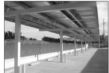
SAMPLE SOLAR CARPOT STRUCTURES
