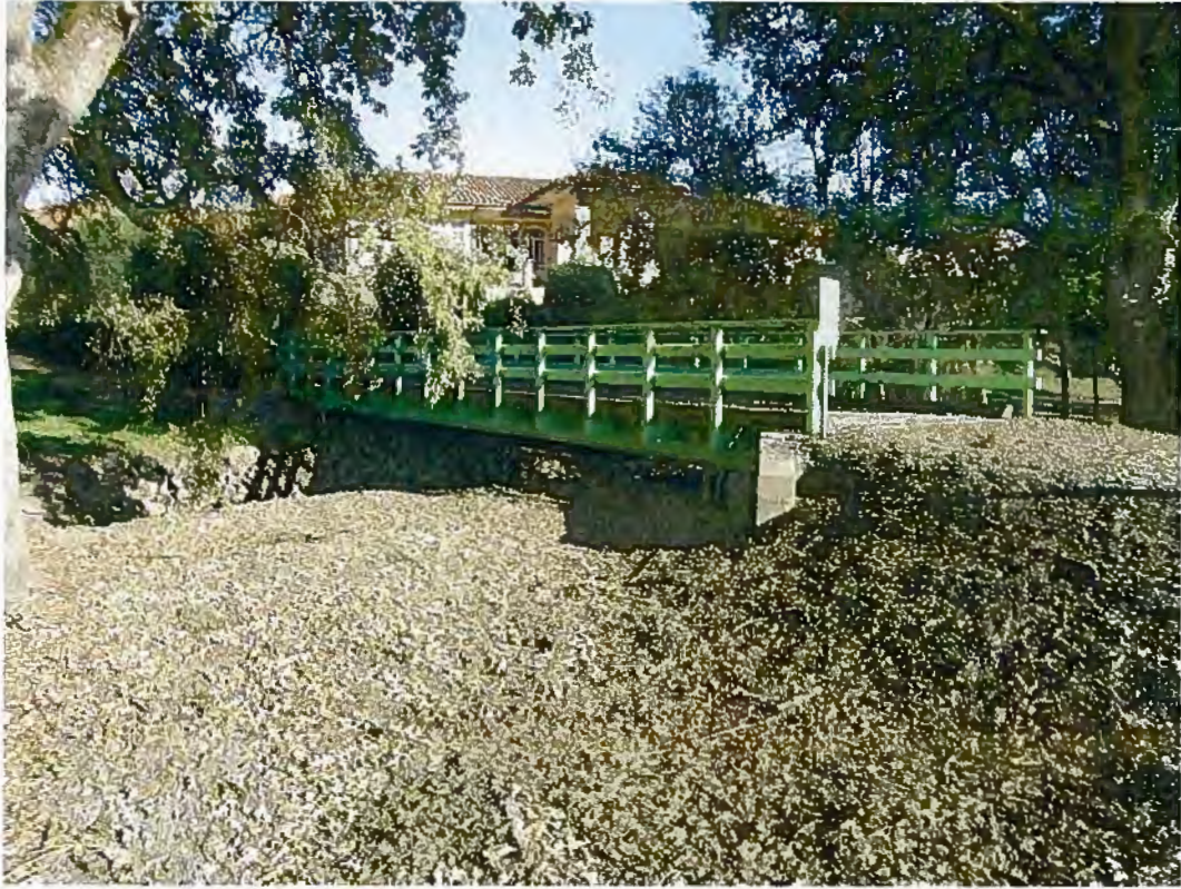
Photo 1. Existing Bridge on property. The project proposes revegetating and expanding the bridge with the construction new footings to accommodate the wider bridge.
