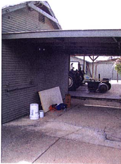
Photograph 13: Southwesterly panoramic view of existing overhang on rear of storage building, May 5, 2010
