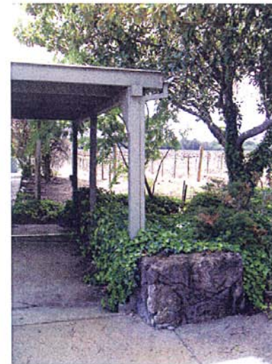
Photograph 12: Southwesterly panoramic view of existing overhang on rear of storage building, May 5, 2010
