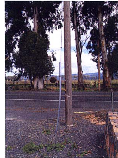
Photograph 23: Northeasterly view of existing power pole at driveway entrance on Cuttings Wharf Road, May 5, 2010
