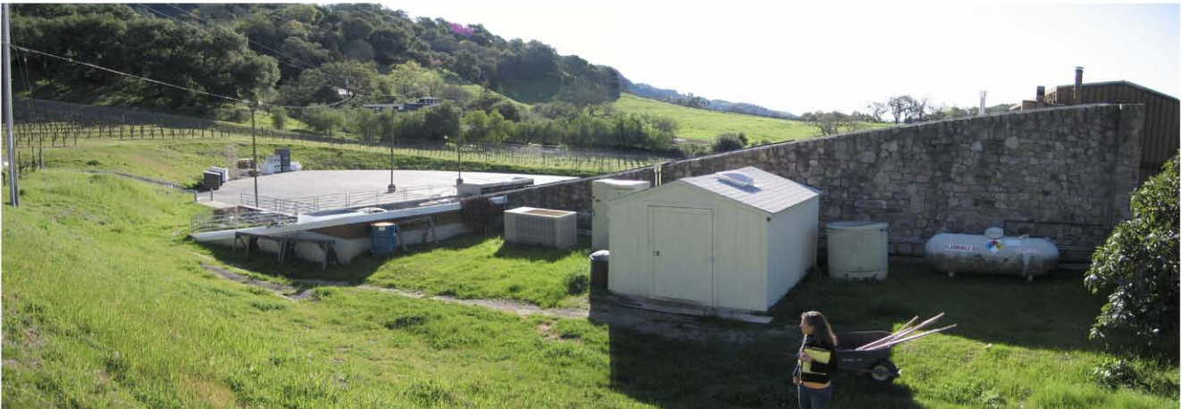
7. View of mechanical area and storage shed, looking Southeast; neighboring field visible in background.
