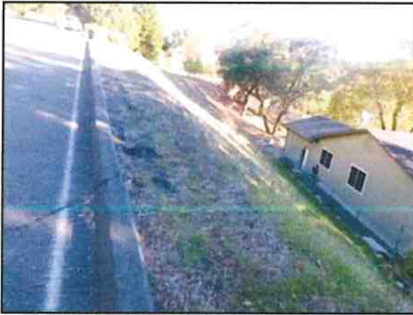
House at 254 Circle Oaks Drive) located below the road. Grading performed during construction of the house caused the road to wash out, requiring extensive repairs, and nearly damaging the home. Again, cracks are visible, indicating more problems ahead for the road.
